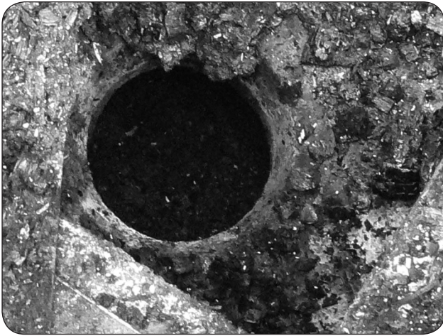
Figure 2. This open pull plug hole is the suspected source of methane from the lower pit that resulted in a nursery barn fire.
