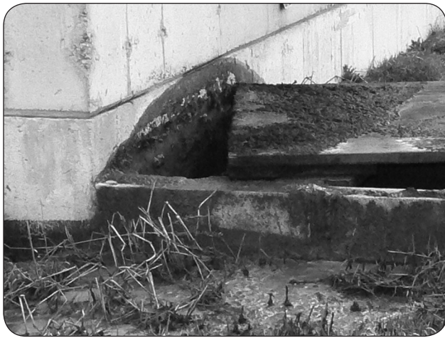
Figure 4. A manure pit cover that was pushed off by manure foam.
